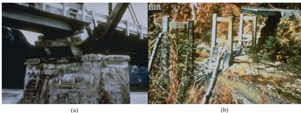
Figure 1. Damaged Bridges: (a) Support damage of the Copper River bridge due to rocking, Alaska 1964 (from USGS Earthquake Hazards Program), and (b) Overturning of three spans of the Agua Caliente Bridge, Guatemala, 1976 (from Public Roads 40(3), pp.101-107, by J.D. Cooper) - reproduced from reference [3]
