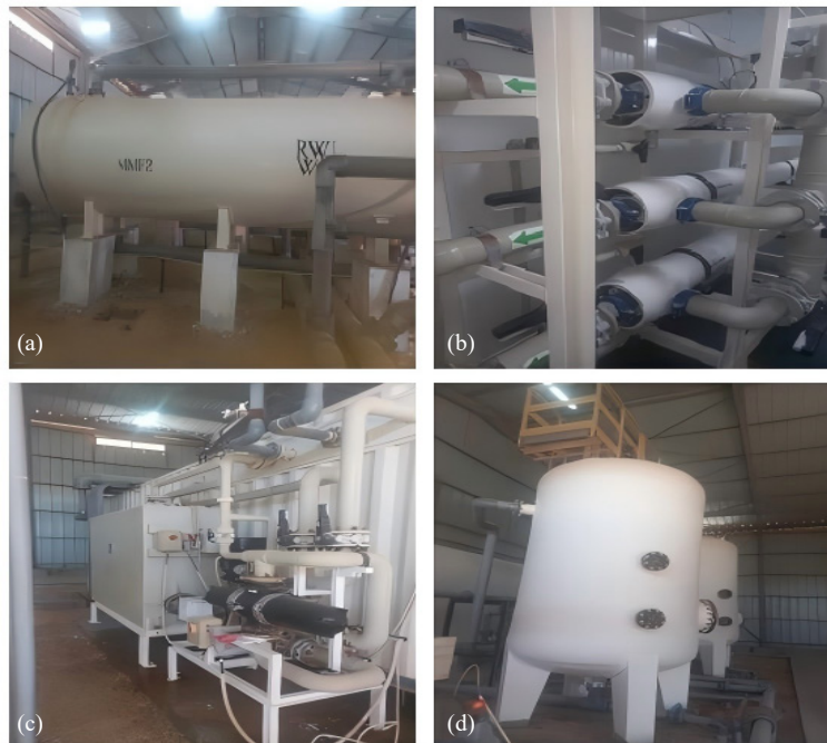
Figure 2. (a) Multi-media filtration units, (b) Cartridge filters, (c) Clean-in-place (CIP) system, (d) Calcite units
