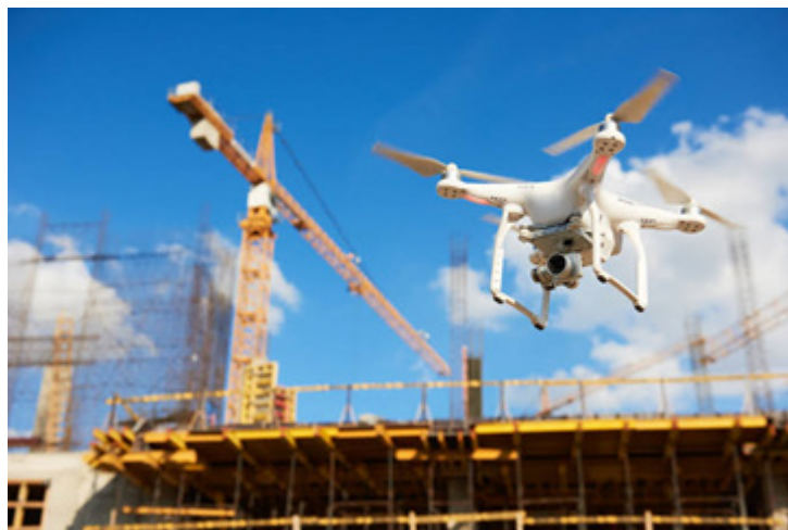
Figure 3. Construction of the Ikeja Bus Rapid Transit (BRT) Terminal with the adoption of drones on a construction site in Ikeja, Lagos State
