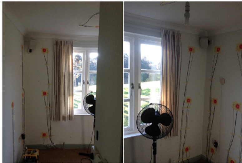
Figure 5. A photograph from test bedroom as it is being prepared for the co-heating test
